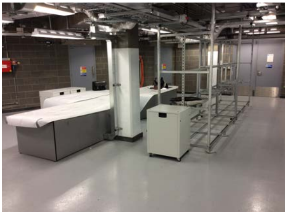
Station operations room test facility at Blackfriars
