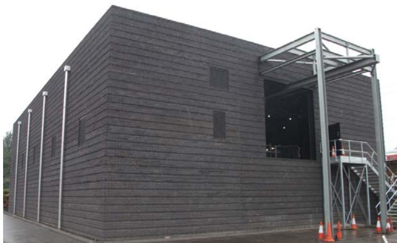
New West Ham high voltage substation
